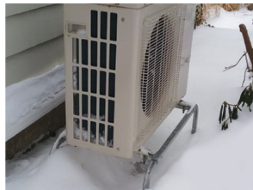
Equipment stand: keeping the unit above the snow (to some degree).
