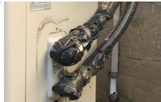
Ensure that the insulation is thorough and covers the entire line set, as shown here.
