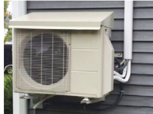
Proper placement: on brackets, insulated tubing, rigid line cover, wind baffle.
